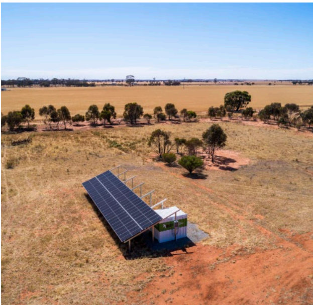
RBSS Power Cube and PV array setup, provides all power needs for the Nangeenan rural home property.
