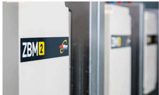
Four x 10kWH Redflow ZBM2 batteries installed.
