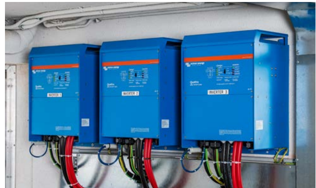
Three x 10kVA Victron Quattro Inverters deliver 3-phase power to the home.
