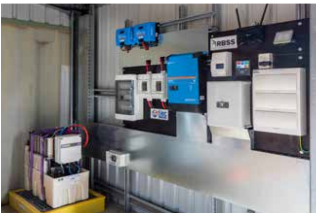
Completed battery room setup - with room to grow
