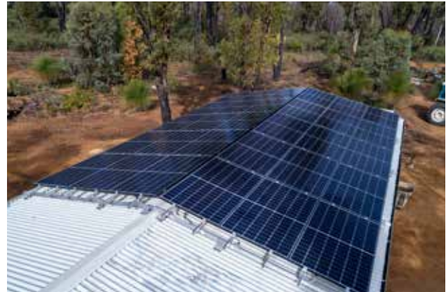
9kW PV array east-west configuration designed to maximise solar yields
