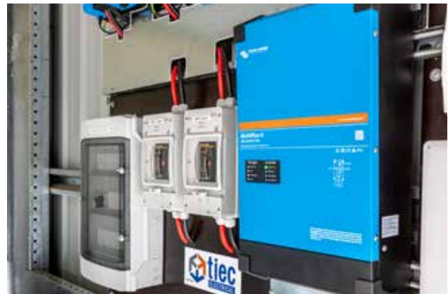
5kVA Victron MultiPlus-II Inverter/Charger, plus PV isolation board and breakers.
